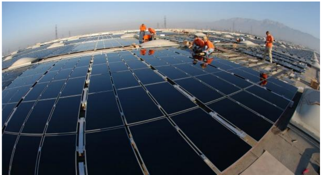
Distributed Rooftop Solar
